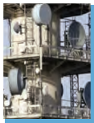
Telecom Data infrastructure
