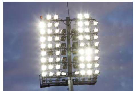
Stadium / Street Road lighting
