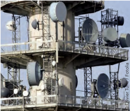
Telecom - Data infrastructure
