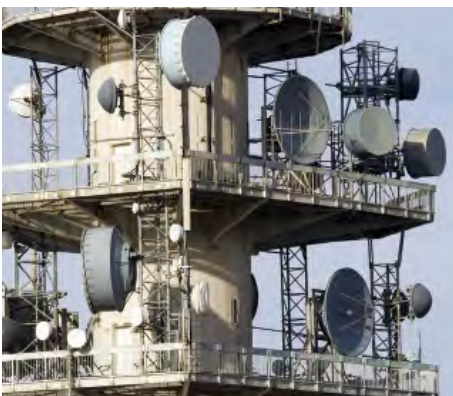
Telecom - Data infrastructure
