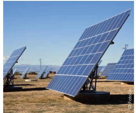
Control Unit / Solar
